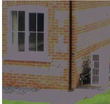
Air source heat pump installation [2]
