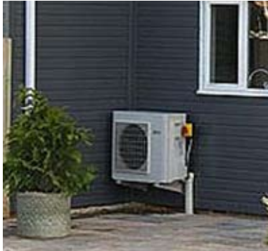
Air source heat pump installation [1]
